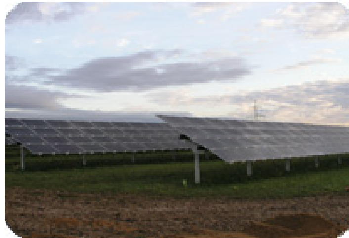
Typical MW-Scale Photovoltaic Installation
