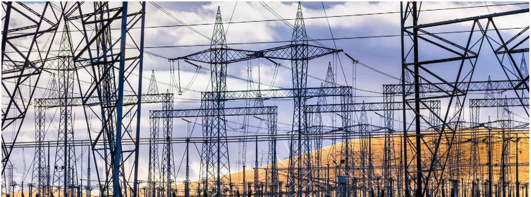
High-voltage electricity towers and power lines at a substation in Central California
