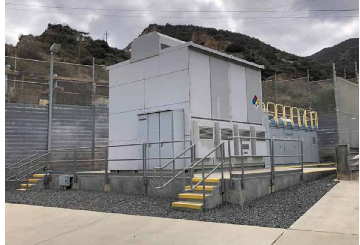
1MW battery storage facility on Catalina Island.
